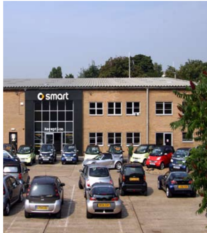
Asbestos roof at London car showroom, repaired and restored using the Kemperol+Coewell system
