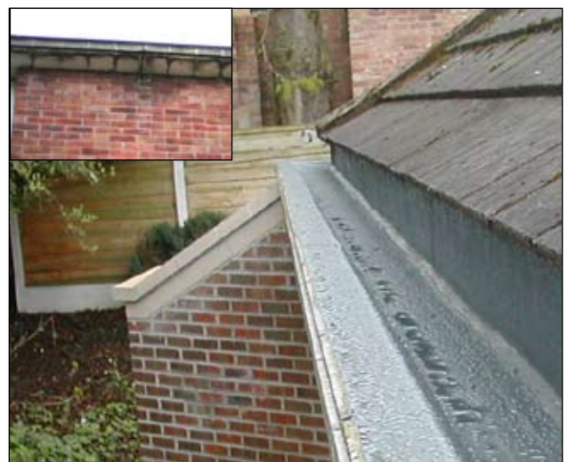
Inset: Typical Finlock gutter failure between adjoining sections
